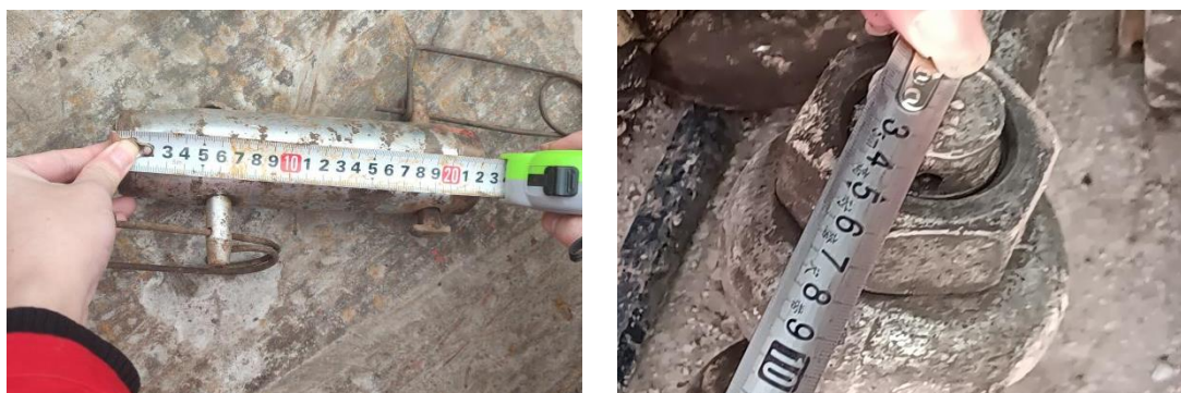
Figure 3.2 Examples of large-size components used at the derrick disassembly and assembly site
